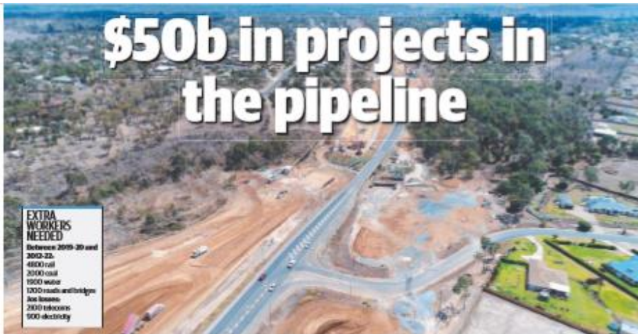
JOB: BOOSE. The Northern Access work progress on Rockhampton's outskirts. The project will link up with the Rockhampton Ring Road, which has been identified as one of the key Queensland projects in the pipeline.
